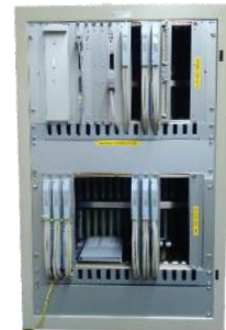
Remote terminal unit
